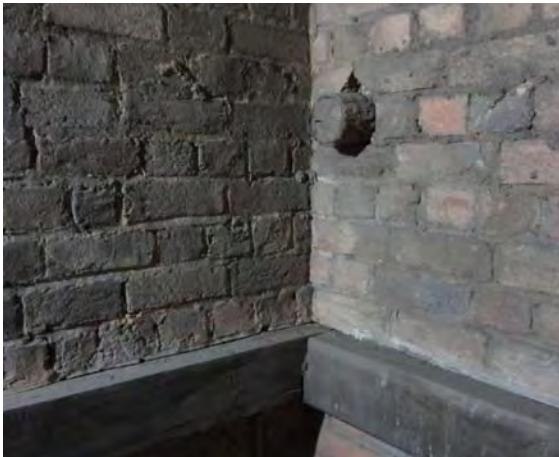
Figure 2.3.49: Remnant of the bush pole scaffolding used to construct the towers remains embedded in the brick walls, North tower.
