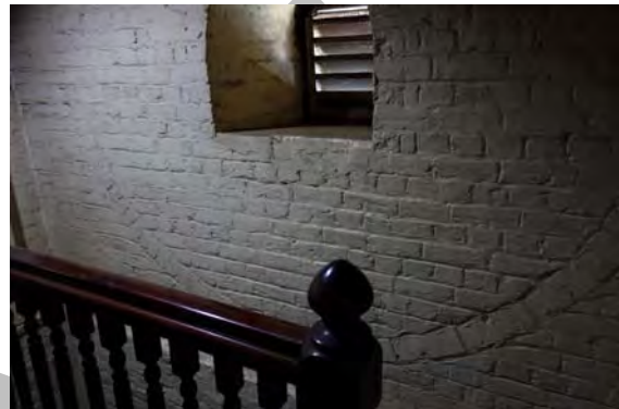
Figure 2.3.41: Inverted brick arch to the brick walls of the tower, inserted as a means to strengthen the tower walls (this photo Level 2, South tower).
