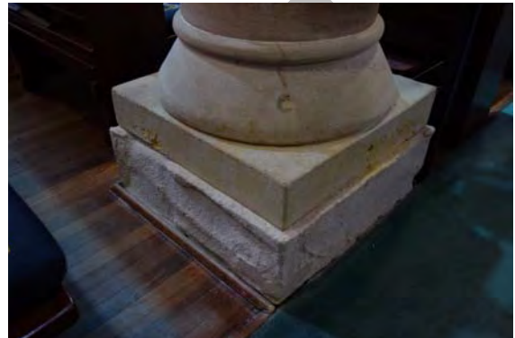
Figure 2.3.56: Erosion of the stone bases would appear to be ongoing.
