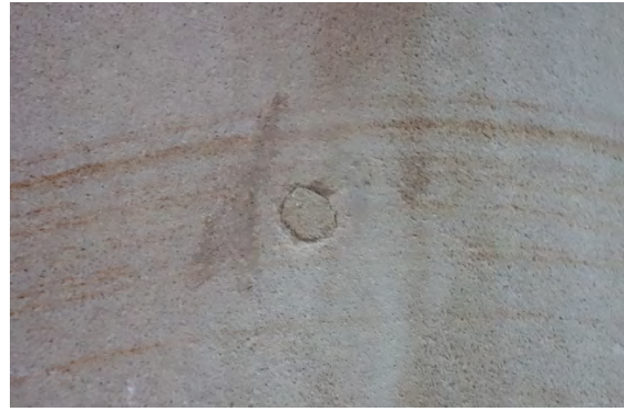
Figure 2.1.37: Evidence in the stone column of the former fixings for earlier kerosene light fitting.
