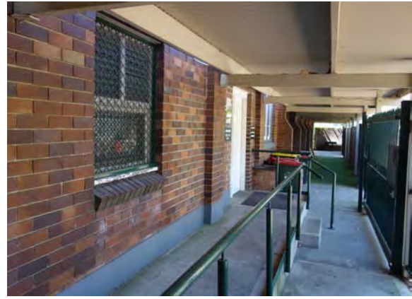
Figure 2.3.68: Timber framed awning extending along the southern elevation of the Parish Hall.
