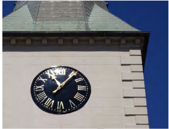
Figure 2.3.23: Thwaites and Reed clock on the northern tower
