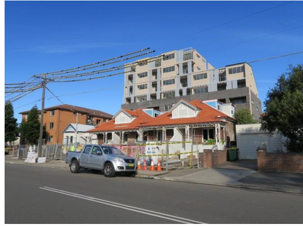
HERITAGE ITEMS AT 17-23 MARION STREET WITH NEW APARTMENT DEVELOPMENT UNDER CONSTRUCTION BEHIND
