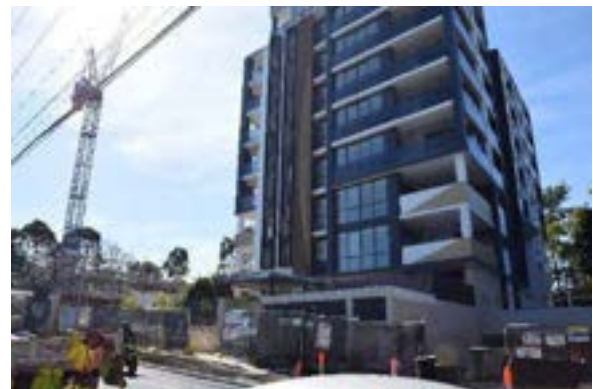
Figure 43. View of the ten storey apartment and construction area adjacent to the site along Shirley Street.
