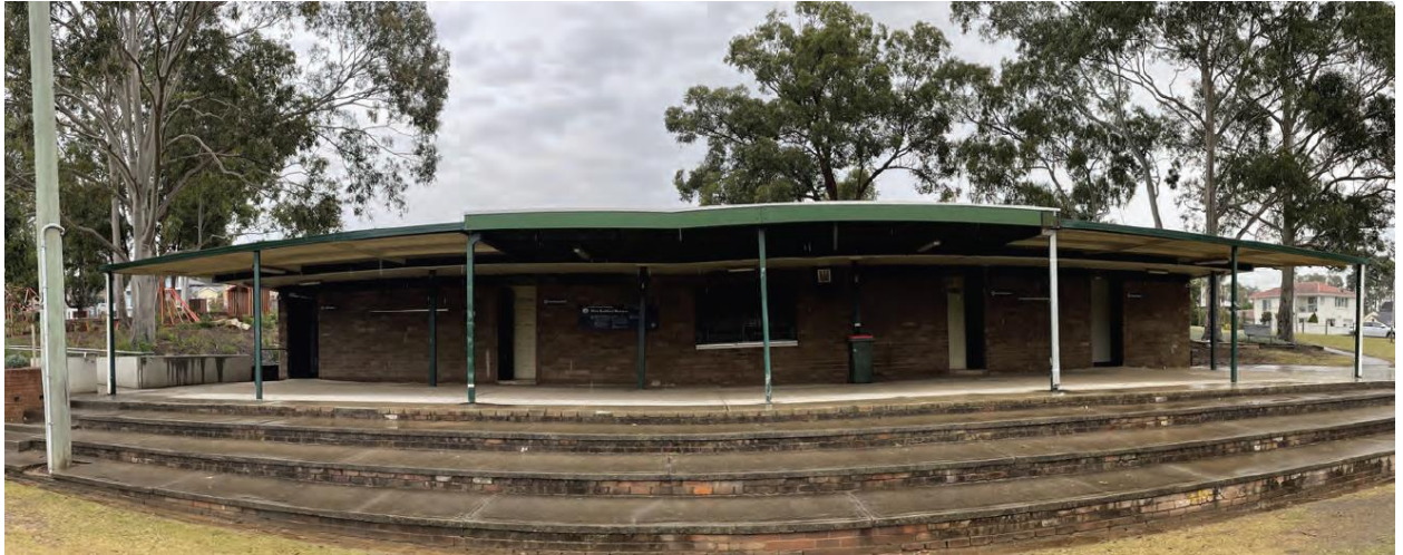
Figure 3 Existing amenities building at Max Ruddock Reserve, front of building looking west (site photos)
