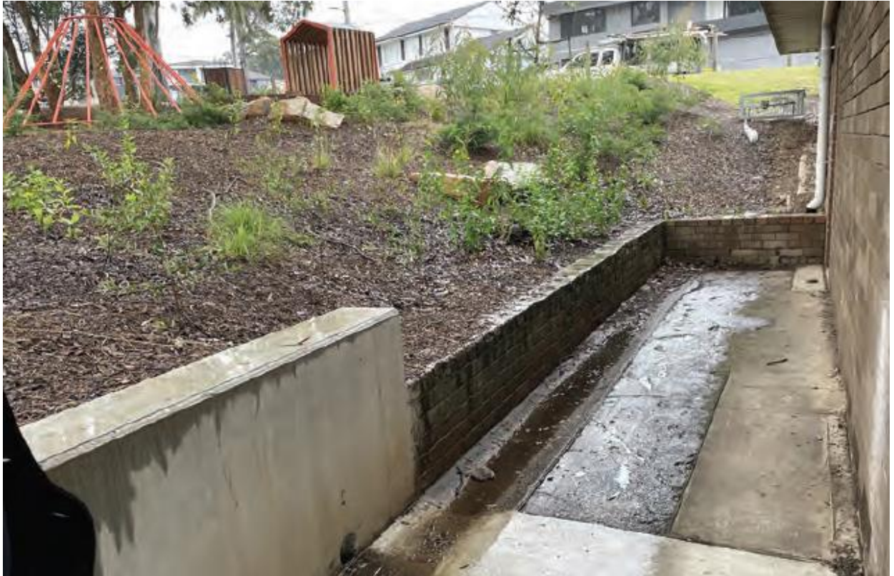
Figure 5 Existing amenities building at Max Ruddock Reserve, rear of building looking south (site photos)
